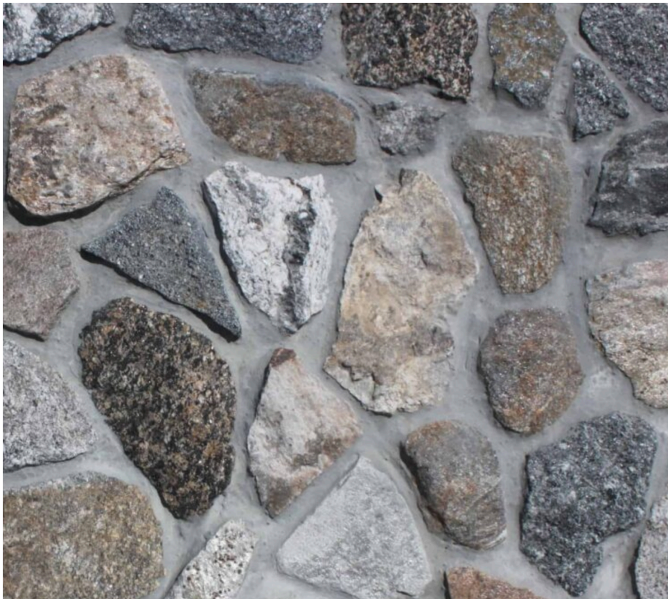
Wide or Over Grout Joint
